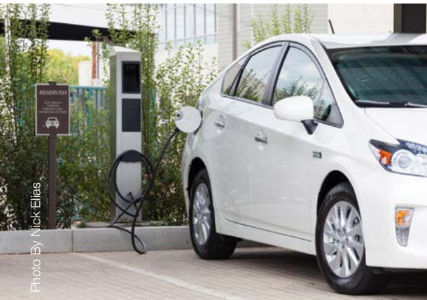
This car charging station at the David and Lucile Packard Foundation is wired by Redwood Electric Group.
