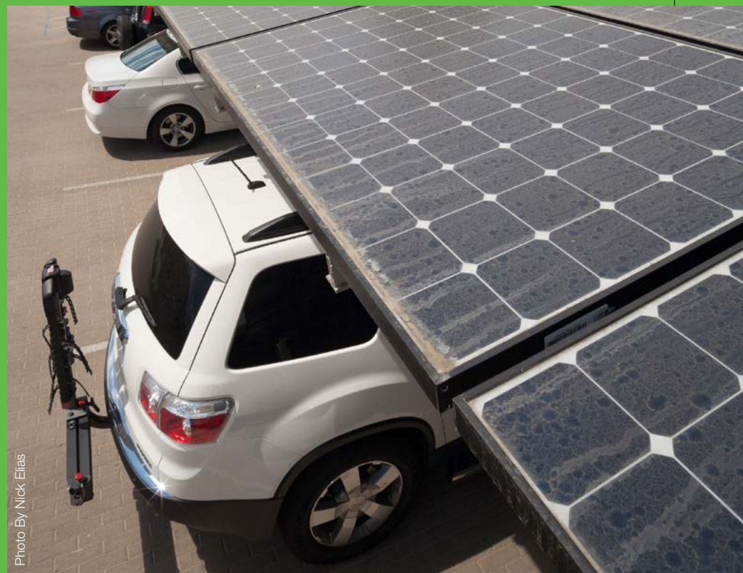
Redwood Electric Group installed part of the photoelectric system on the roof of the parking garage.
