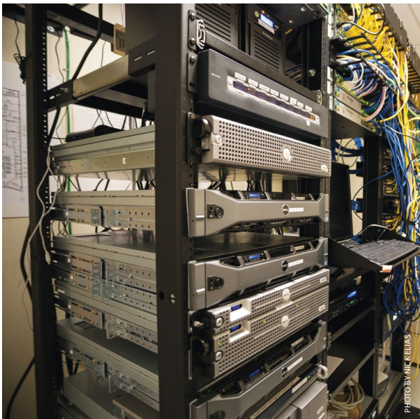
Paganini Communications wired the third floor server room, along with its central monitoring station inside the third floor server room.
