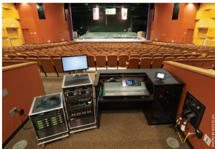
The center mix position, located in the middle of the auditorium, holds a state-of-the-art Yamaha LS9 digital mixing console that controls the sound system. It was installed by Lloyd F. McKinney Associates.
