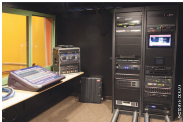
The Capuchino Theater control room includes equipment for lighting control, video projection, amplification, TV channel distribution and the intercom system.
