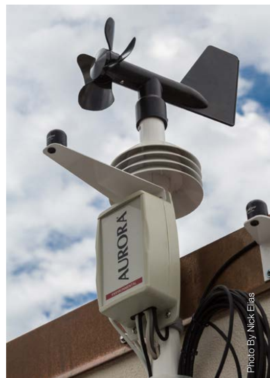
Redwood Electric Group wired the weather station on top of the facility.
